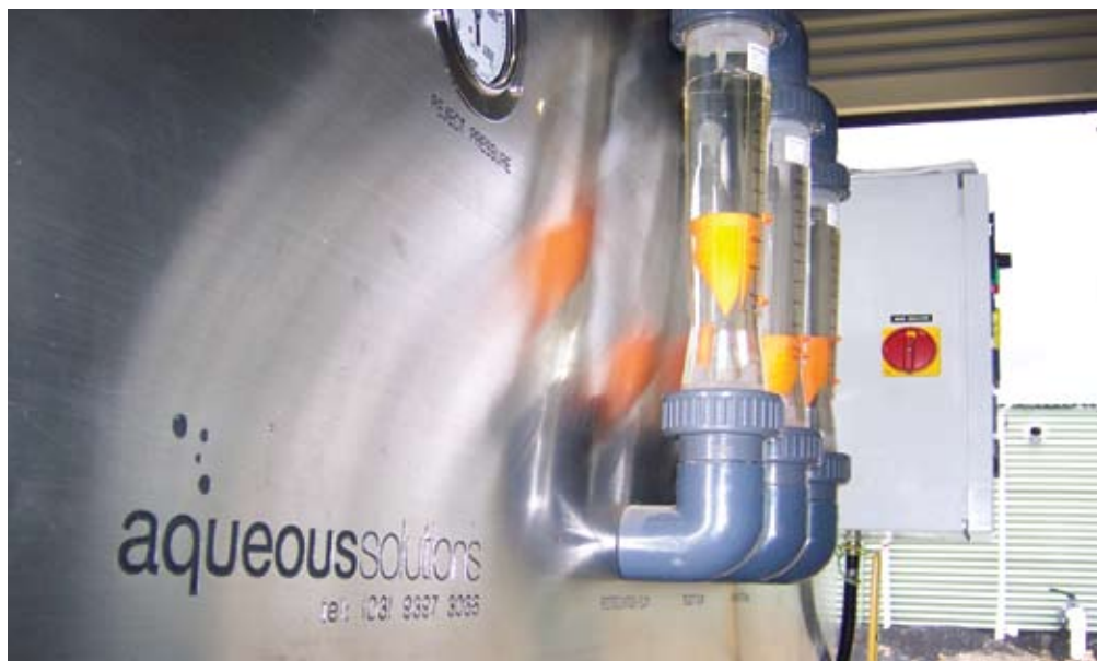
Desalination Plant at Wesley College by Aqueous Solutions.
